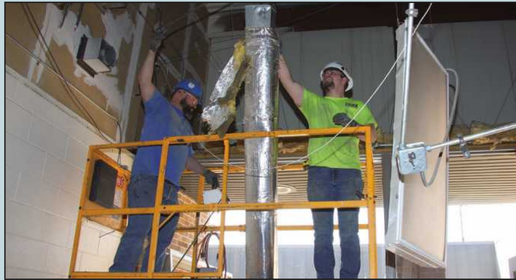
SETTING DUCTWORK at the Jacobetti Complex at Northern Michigan University in Marquette are (l-r) Jesse Anderson and Dustin Lohfink. The Sheet Metal Workers Local 7 members are employed by Dresseler Mechanical Inc.
