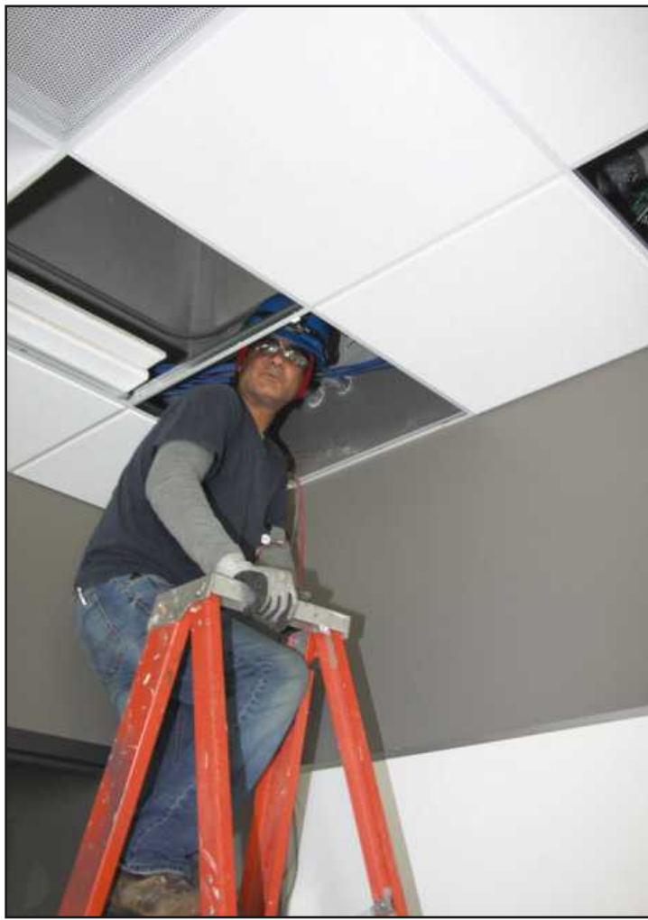
ELECTRICAL WORKER Will Choudhry peers above a drop ceiling before installing a fixture at the Jacobetti Complex renovation project at NMU in Marquette. The IBEW Local 906 member is employed by S&T Electrical. Photo credit: Jack Deo
